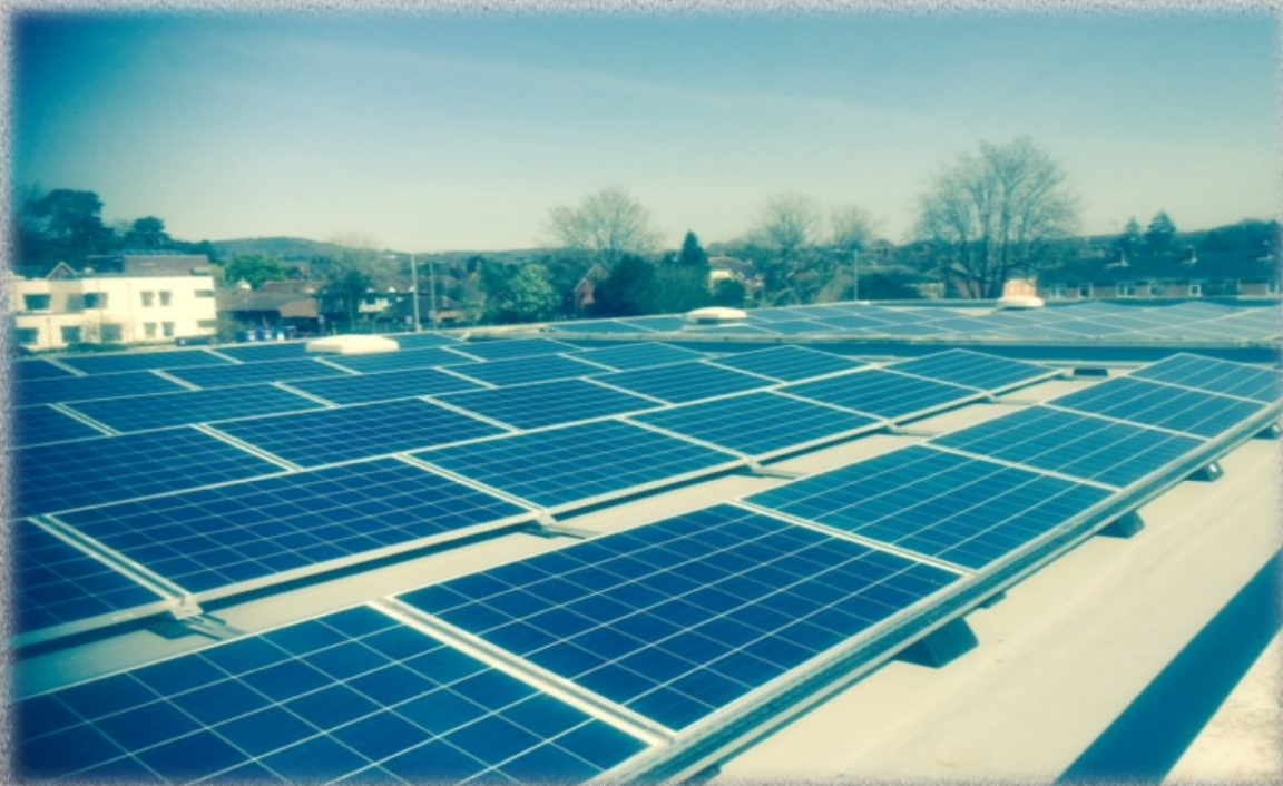
PV array at Cranleigh Leisure Centre
